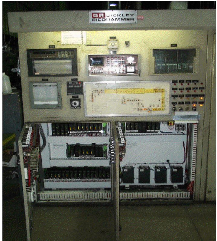
Control Cabinet – After Upgrade
